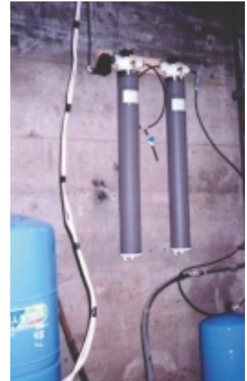
POU installation for household kitchen sink using adsorptive media. Device located in the basement of a household in Maine.
