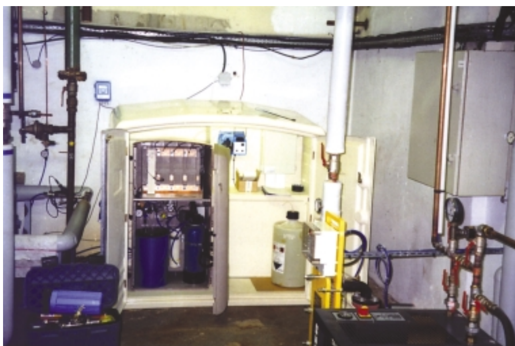
Alternative treatment to highly corrosive chlorine makes use of the complementary and alternative activity of two organic nonoxidizing biocides that attack both the Legionella organisms and their nutritive environment—biofilm.
