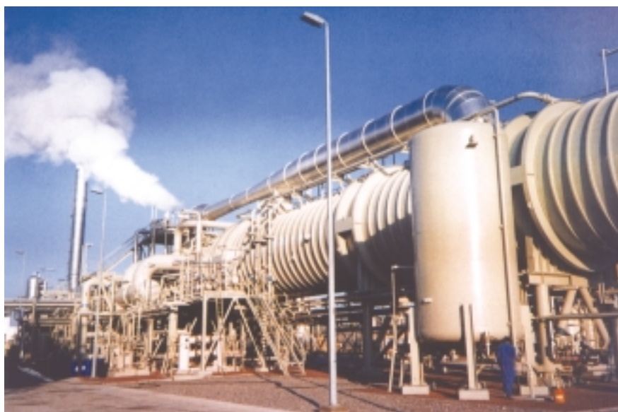
This multiple-effect vapor compression distillation system is in operation in Abu Dhabi in the Middle East. Many similar units are being installed across the United States to produce drinking water from sea water.
