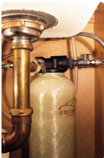
An under the sink, cold-water tap, point-of-use arsenic removal system.
