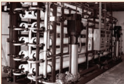
A dual RO system installed at Jupiter Island Golf Club.
