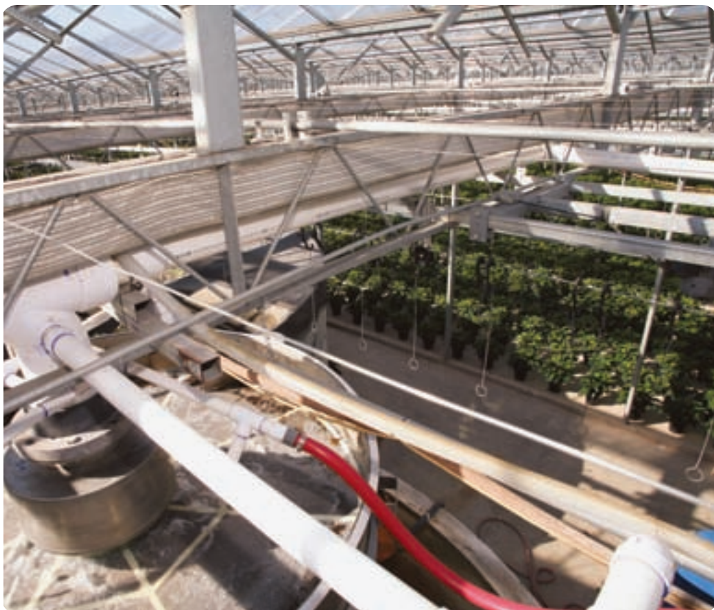
Leaves, peat moss and other debris are screened from up to 500,000 gal of water per day at this nine-acre greenhouse.
