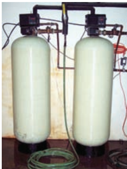
The unit had to be set up as a twin system with a System 9 configuration, allowing for a 40 gpm flow rate and continuous soft water.
