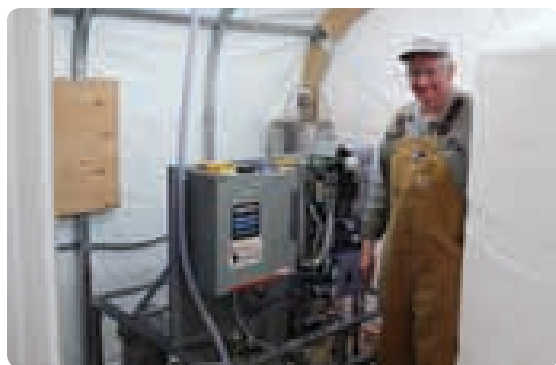
Jon Dufendach approves a new 5 gpm filtration/ozonation plant at a central Alaska mining exploration camp.
