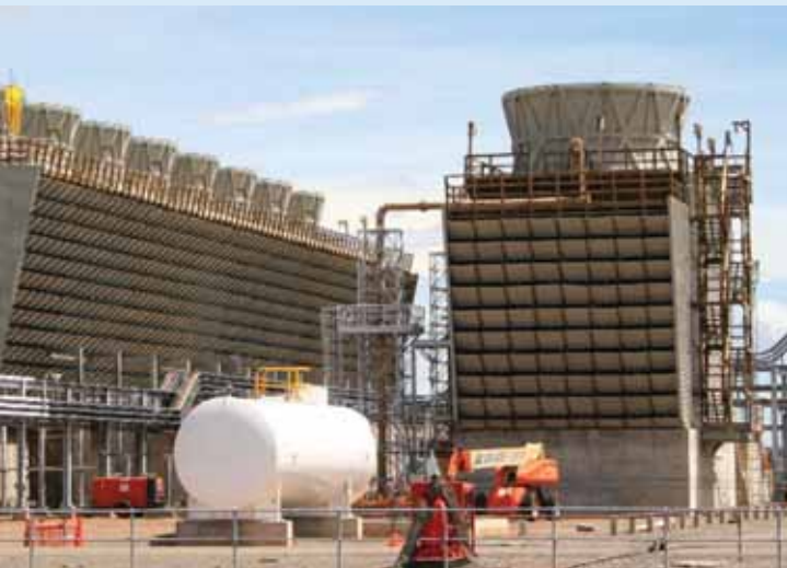
Improving filtration for cooling water represents a tremendous opportunity to reduce energy, chemical and water use.
