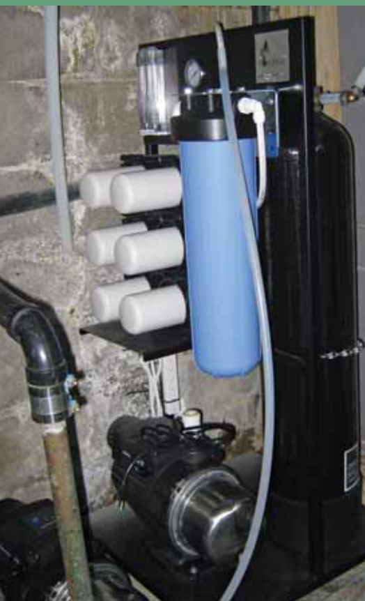
Lord Fletcher's installed more efficient softeners and a central RO system.
