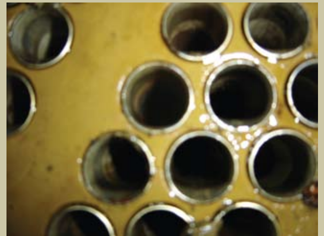
A main condenser tube sheet after extended run in a NIPSCO power plant before cleaning, after 2.5 months of MIOX treatment.
