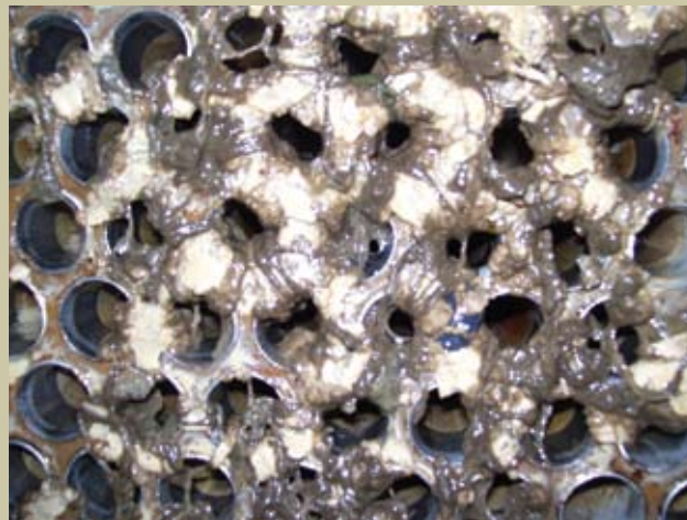
A main condenser tube sheet after extended run in a NIPSCO power plant before cleaning, after non-MIOX treatment.
