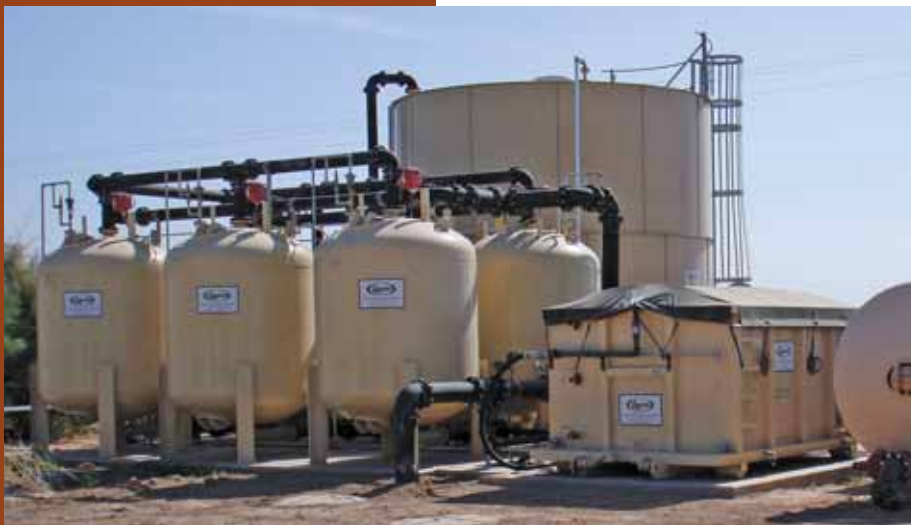
A CF arsenic removal system at Casa Grande, Ariz., designed to treat a flow rate of up to 1,350 gpm.
