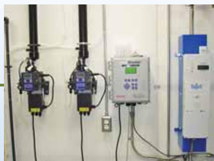
Bottom: The systems have multiple built-in redundancies. This increases security and provides educational opportunities without having to shut down the entire system.
