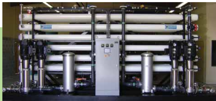
This 500,000-gpd RO system succeeded in substantially reducing sodium and chloride levels in Spirit Hollow's water.
