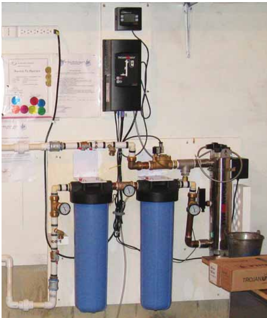
The North Boswell Water Users Community uses a Trojan UV Max Pro 10 system with 1-micron absolute filtration to meet drinking water standards.
