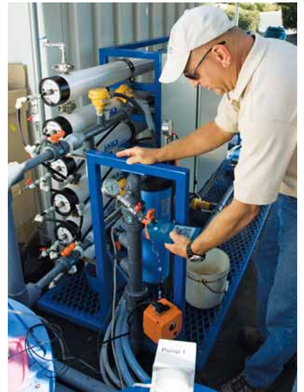
A staff member tests influent ORP at an RO desalination plant. Some manufacturers of disinfectant-sensitive equipment provide ORP tolerance values for prescreening and influent control.
