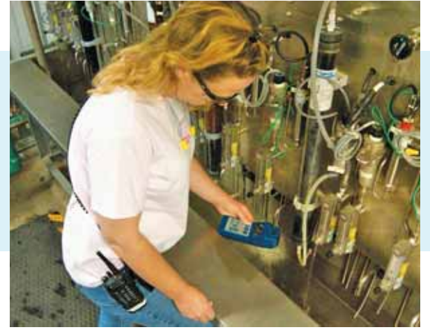
At the same power plant, the staff member measures ORP in water from a cooling tower control panel.
