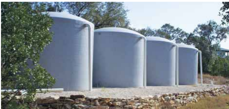
The 20,000-gal tank farm is hidden from the house by a stand of oak trees.
