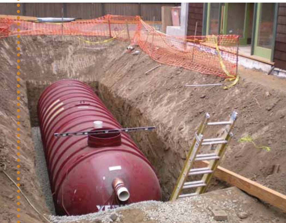
An underground rainwater cistern is installed in a California home's backyard. (Photos courtesy of Neal Shapiro, city of Santa Monica, Calif.)
