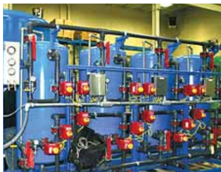
The system treats water to meet local discharge requirements for iron and manganese.
