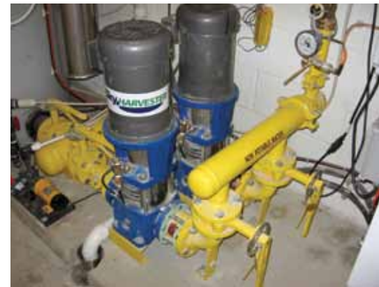
Booster pumps supply harvested rainwater to the non-potable water plumbing system for toilet flushing.
