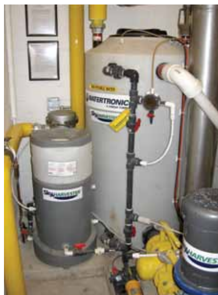
The disinfection system includes a 50- \mu bag filter (background), tablet chlorination system (foreground) and day tank.
