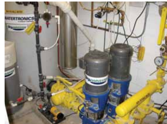
The chlorination system, day tank, booster pumps and chlorine analyzer (mounted on the wall) provide treatment for the rainwater.
