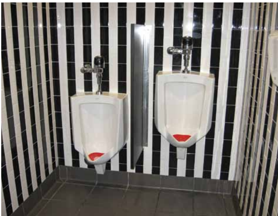
The toilets and urinals in the park's restrooms are flushed with harvested rainwater.
