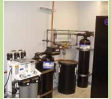
Location: Universal City, Calif. Size: 4.5 gpm Cost: $65,000+ Contractor: Eversoft Inc.
