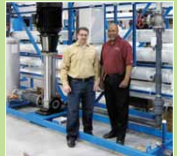
Location: Savannah, Ga. Size: 800 gpm Designer: WaterProfessionals Owner: U.S. Army Corps of Engineers
