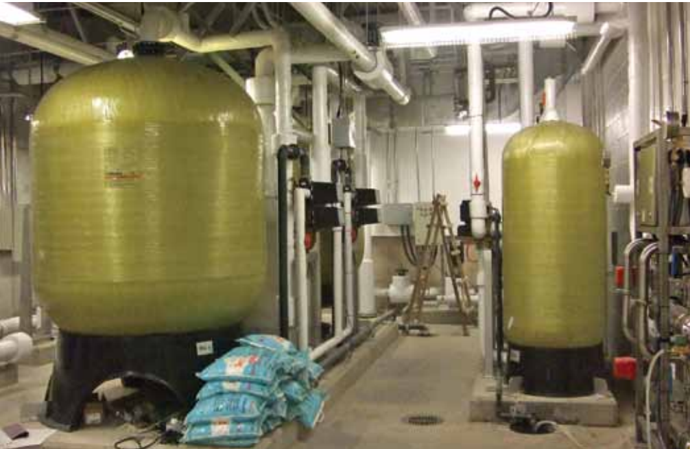
Tank-type systems, like this one at the U.S. Consulate in Beijing, include carbon, iron, sand and multimedia filters, along with softeners, de-alkalizing systems, acid neutralizers and specialty contaminant removal systems.
