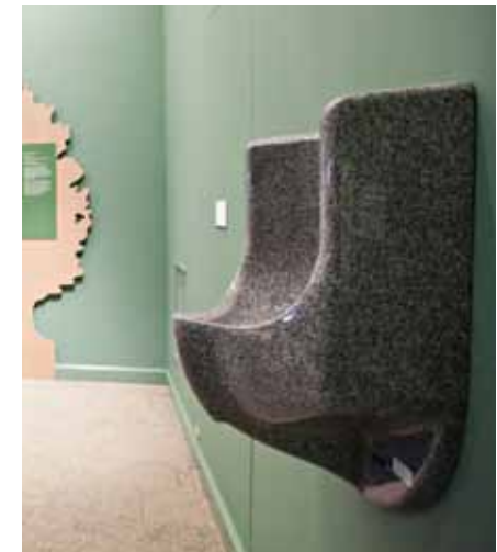
Each waterless urinal, like this one, installed in a green school can save a facility up to 40,000 gal of water per year.
