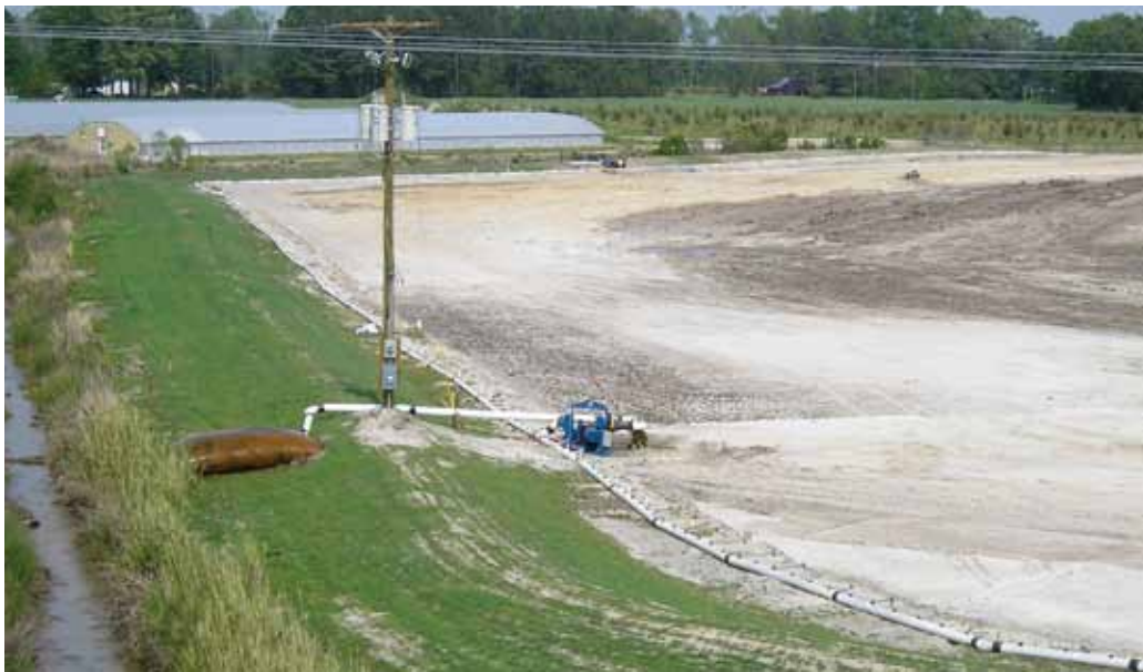
Above: Two different views of wellpoint dewatering systems with filter bags, which trap suspended solids, allowing clean water to discharge into the environment Opposite: A pump and stripping system, often used for applications such as groundwater containing oil or gas
