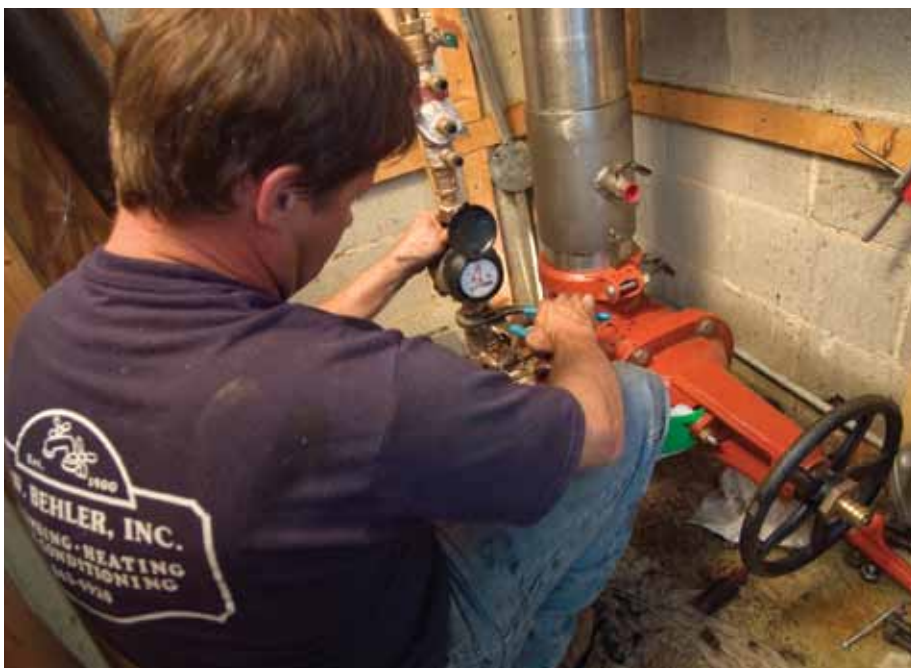
An F.W. Behler technician installs the water meter on a DCVA fire line backflow preventer.
