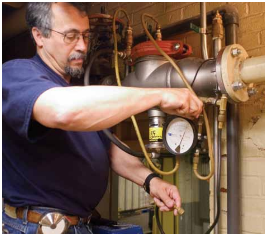
Yates double checks the differential pressure for the first check on an RP serving a glycol-infused loading dock sprinkler system.
